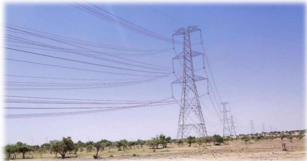
New high voltage powerlines are coming up despite stay order by National Green Tribunal © Sujit Narwade
